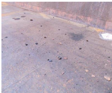
Not grain clean – loose rust and debris on tank top
