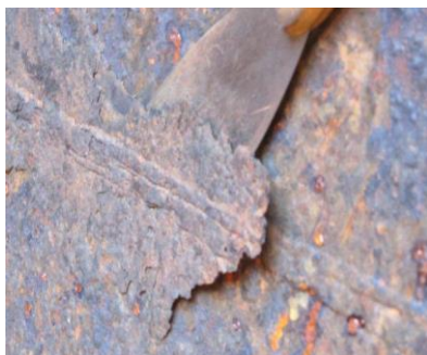
Not grain clean – loose rust found by surveyor
