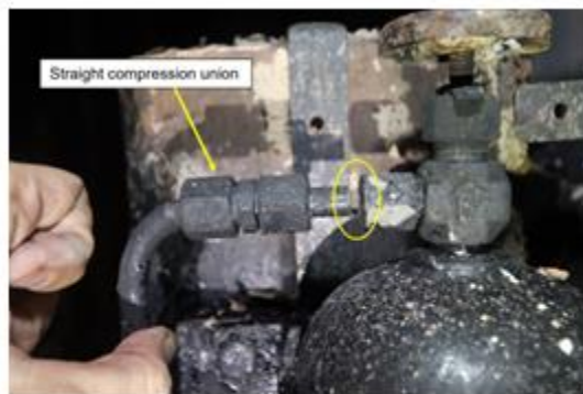
Fractured copper pipe
