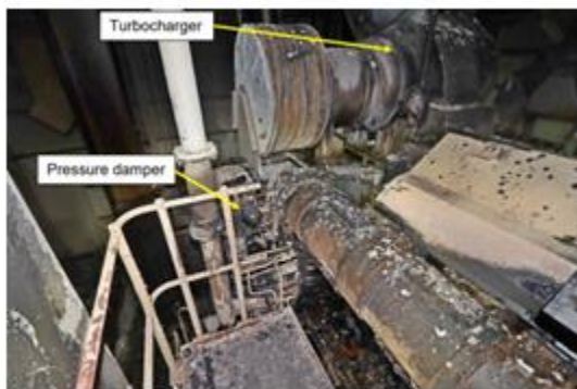
Fire damaged area of auxiliary engine
