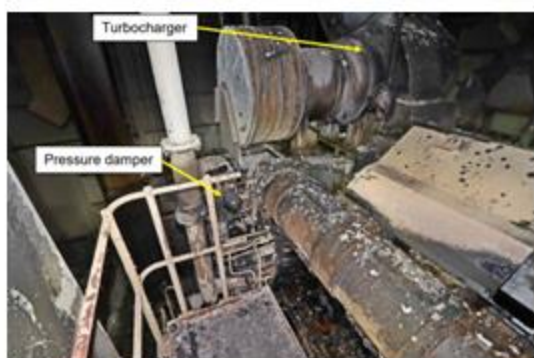
Fire damaged area of auxiliary engine
