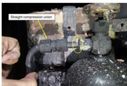
Fractured copper pipe
